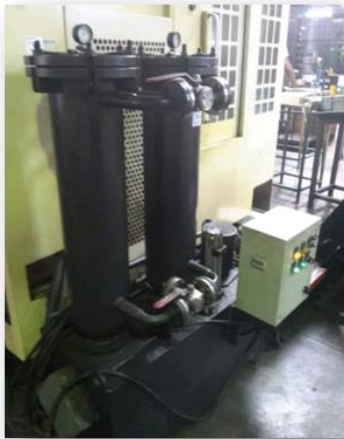
Fig 3. Oil contamination filter
