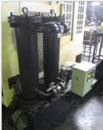
Fig 3. Oil contamination filter
